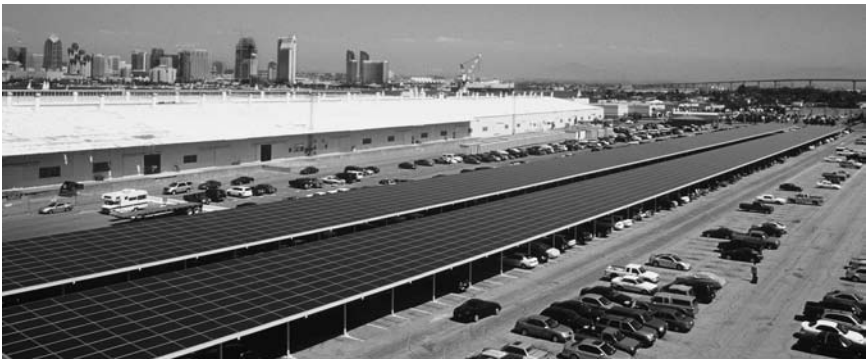
Figure 3-5: U.S. Navy 750 kW Parking Lot Solar PV Installation Near San Diego
