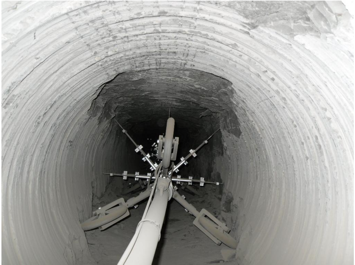
Figure 6.1: Squaring of a horizontal borehole in ANDRA's underground laboratory at Bure. (Photo credit: Krishan Wahi, 18 August 2010)
