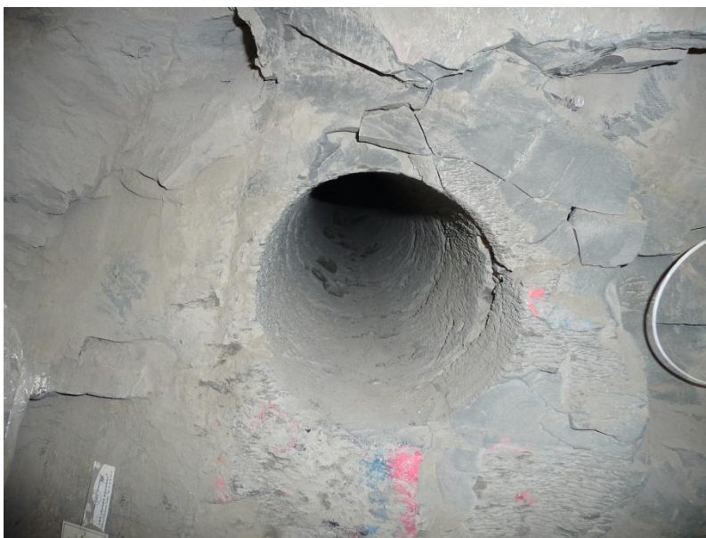
Figure 4.1. Fractures around a borehole drilled from a Bure laboratory gallery (Photograph by Arjun Makhijani, August 18, 2010. P1020429).
