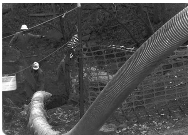
Workers vacuuming sediment out of Acid Canyon, Los Alamos National Laboratory, November 2001.
